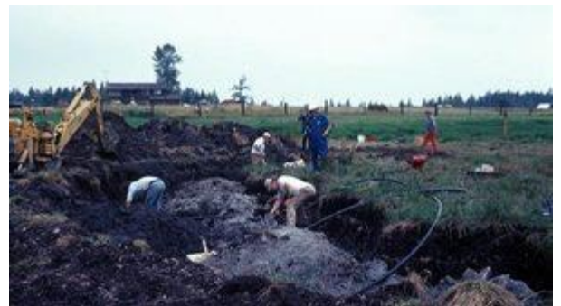
This photo shows the first day of excavation work on the site in Sequim in 1977 (The Seattle Times).
